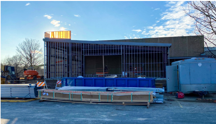
Progress continues on the Theater Renaissance project. Workers have started building the frame and the roof of the new addition to the Zwermann Arts Center.
