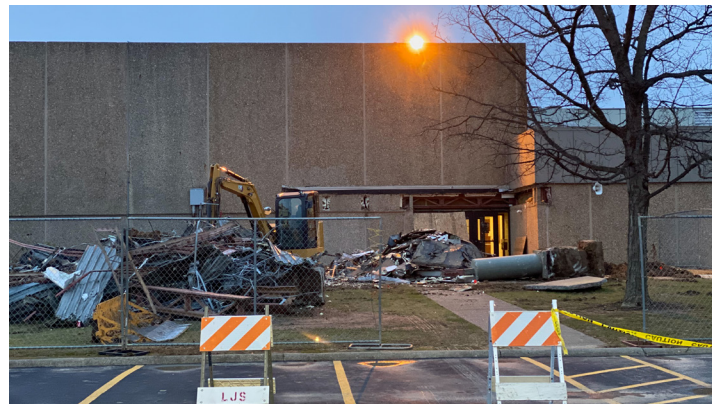
The east awning of the Performing Arts Center is removed on the first day of demolition of the Theater Renaissance project.
