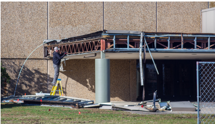
A worker begins the demolition on the Performing Arts Center to prepare for the Theater Renaissance construction project.
