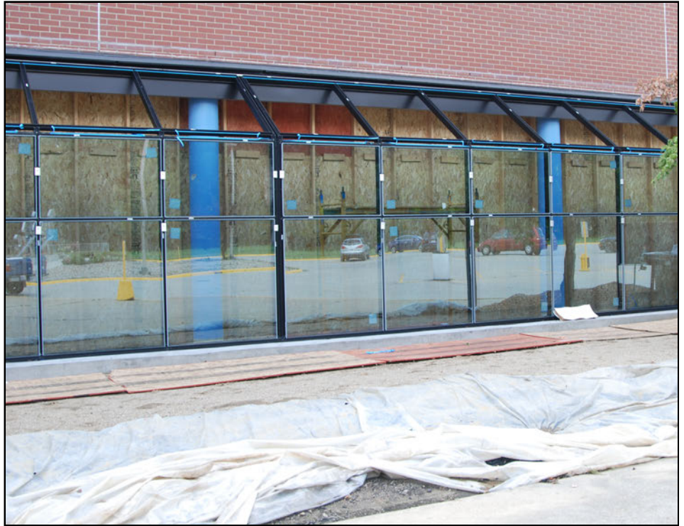
Renovations have been underway this summer on the atrium in the Dr. John D. Stull Performing Arts Center. The work included replacing the original glass and floor tiles.
