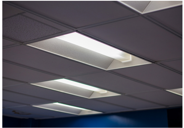
Approximately 2000 lights in Williams Hall were upgraded to new LED fixtures at no charge. O&M Team Leader Chris Ellington found the deal for the labor and materials for the project.
