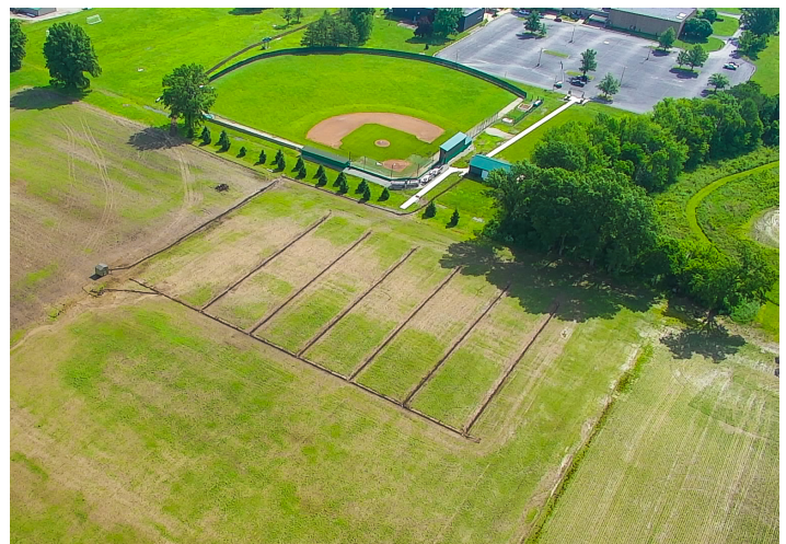
Once the irrigation work is completed field work will begin to build the competition field and the practice field to prepare them for the fall season.
