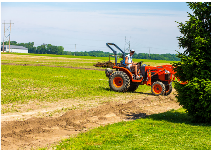
A contractor digs trenches as work gets underway to install irrigation at Statesmen Park.
