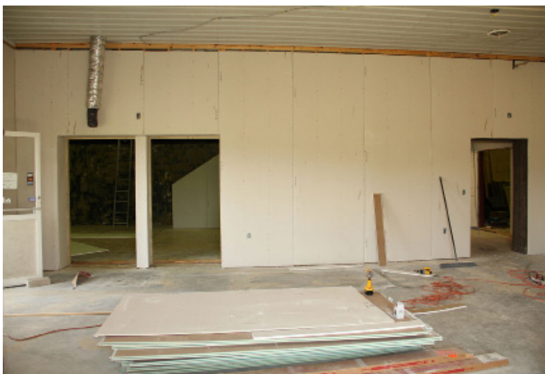
Drywall is going up in the Bobcat Coffeehouse. A doorway has been cut that leads into the student lounge (pictured right).
